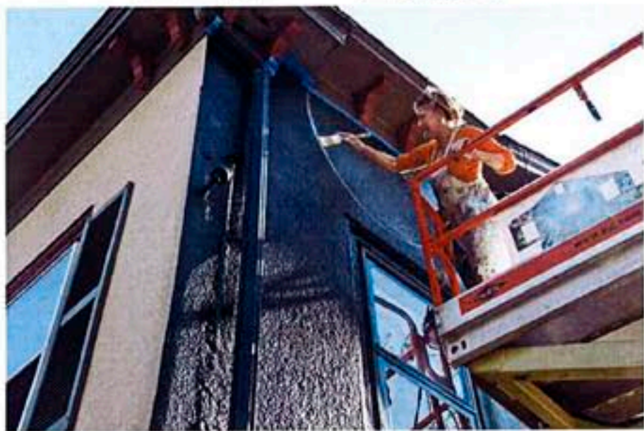
Muralist Ilia Berger, up on a scissor lift, paints the wall of Witherspoon Bread Company. (Photo courtesy Terra Momo Bread Company)
